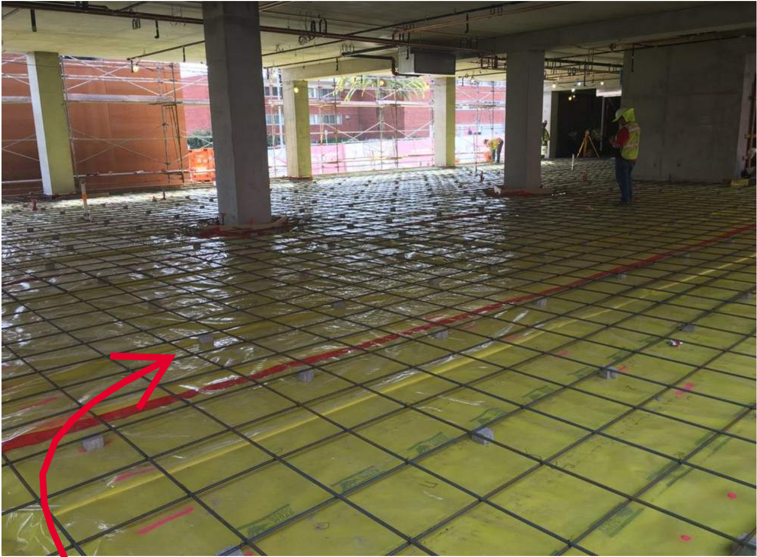
REMAINDER OF STUDENT SUCCESS BUILDING LEVEL 1 - SLAB ON GRADE - IS BEING PREPARED FOR PLACEMENT!
