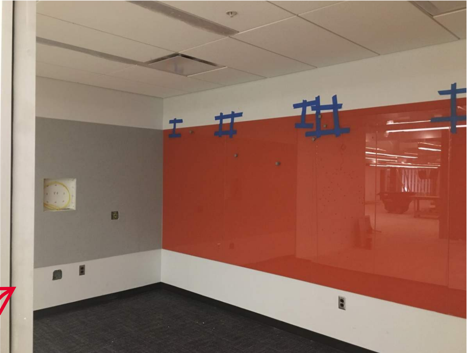
MAIN LIBRARY POD 'A' LEVEL ONE STUDY ROOM MARKERBOARDS AND SOUND ABSORPTION PANELS ARE INSTALLED
