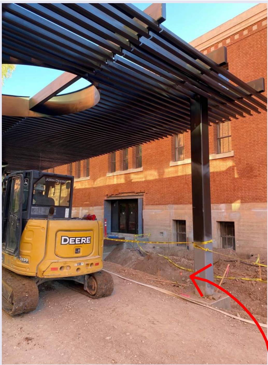
On the left the historic gym floor has been sanded and the basketball lines have been painted. On the right the steel shade canopy is being painted and the doors leading to the Albert B. Weaver Science and Engineering Library are installed. Check it out!
