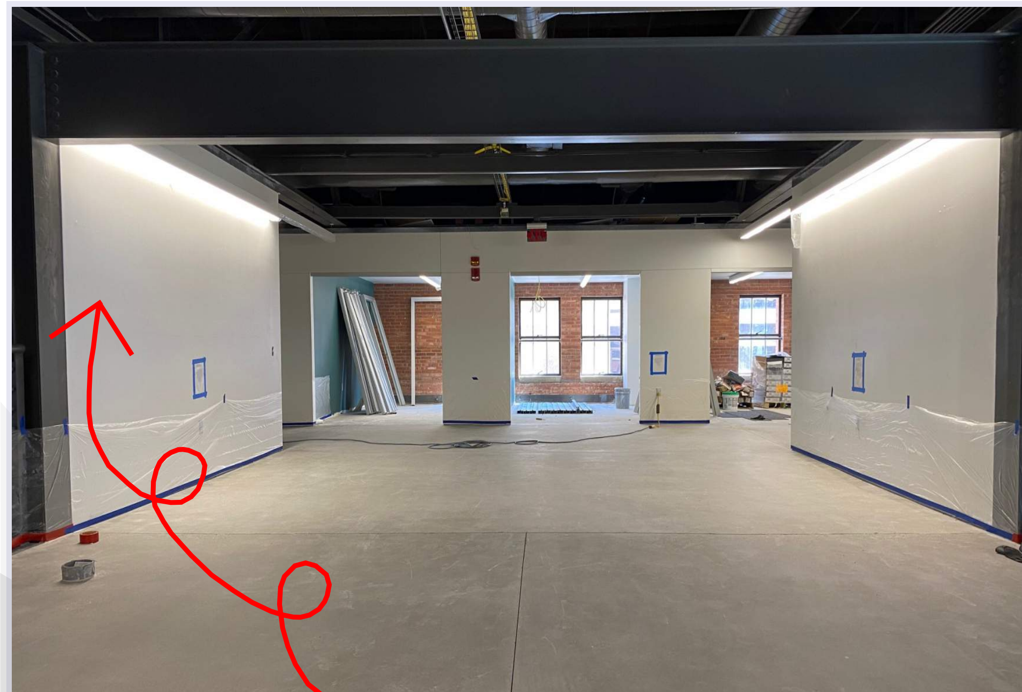
On level 3, light fixtures have been installed in the corridors and conference rooms! The concrete floors on level 3 are also being polished this week.
