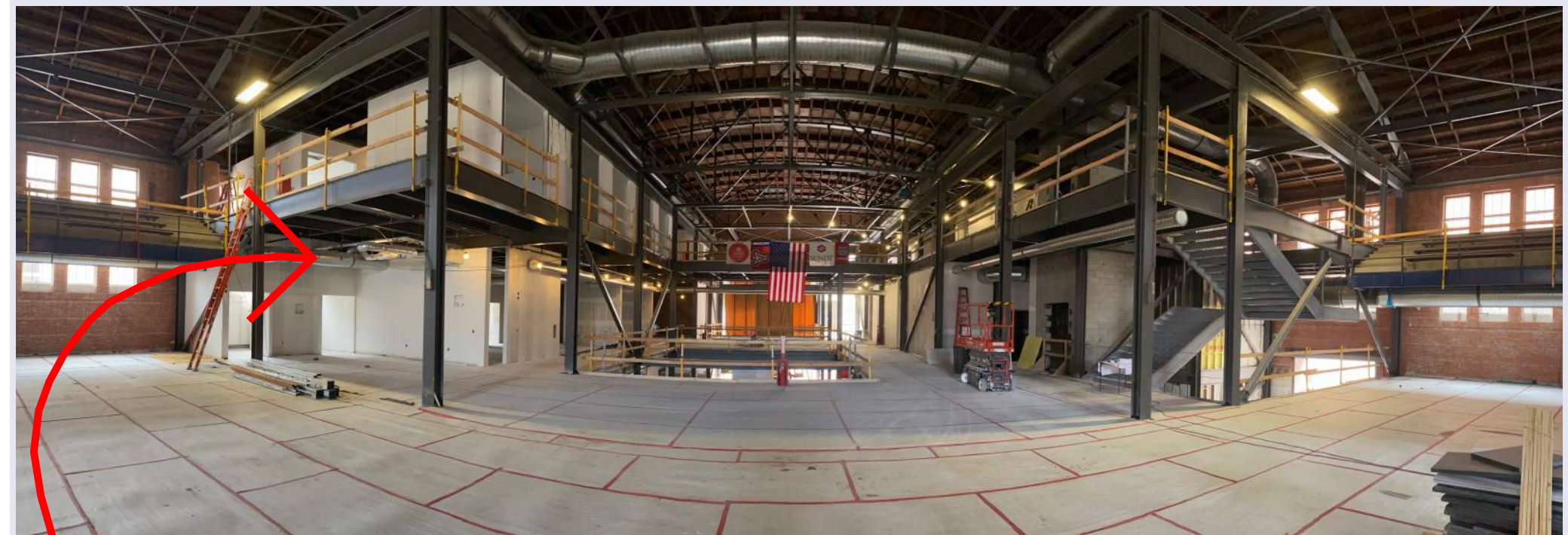
Inside the main entrance standing on the historic gym floor, looking south. Level 3 bathrooms are getting tile! Level 2 is getting paint, and level 1 is getting framed and drywalled!
